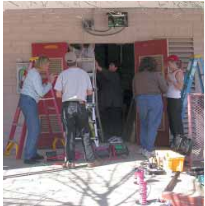
Instructor Carol Weis (in red baseball cap) oversees the construction of the complicated junction box, affectionately dubbed the "artificial heart."
